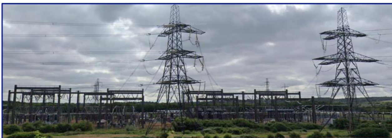
Image 4.4 Illustrative example of a typical AIS substation
